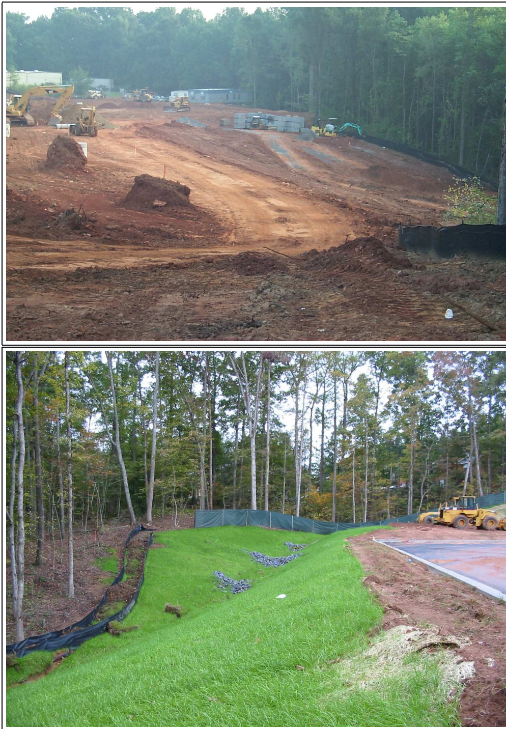
Figure 2.2: Example of spatial construction where a large area has been cleared prior to development. Upper photograph taken before erosion and sediment control measures have been installed. Lower photograph taken after installation of erosion and sediment control measures.
