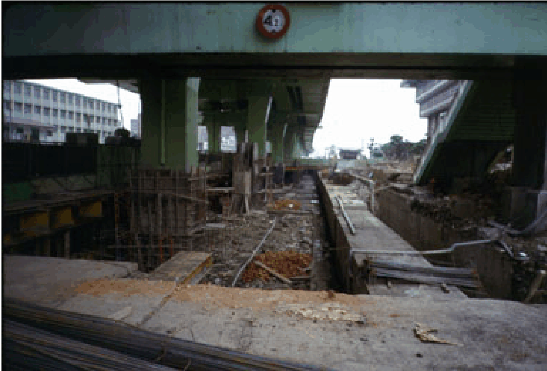
Figure 3-5: This is one of many construction sites in support of Taipei's new subway system (now completed). This site, adjacent to Taipei's main rail station, is typical of the 3-D jobs (dirty, dangerous and demanding) and worksites in which overseas contract laborers from Thailand were obliged to work.
