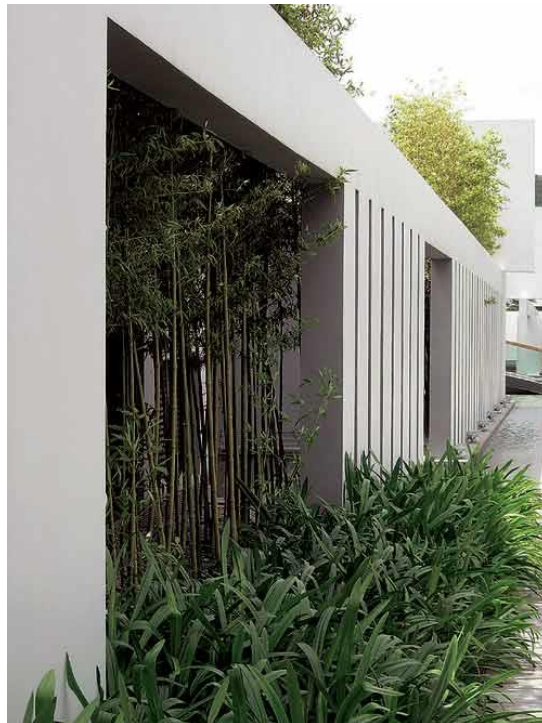
Figure 4.7 A View of Leaking through Scenery
