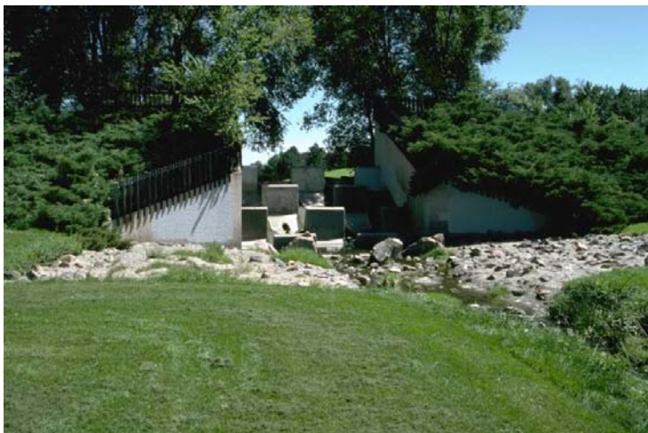
Figure 3.13 Hydraulic structure blended into the landscape, Colorado (Urban Drainage Criteria Manual, 2001, HS-7)
