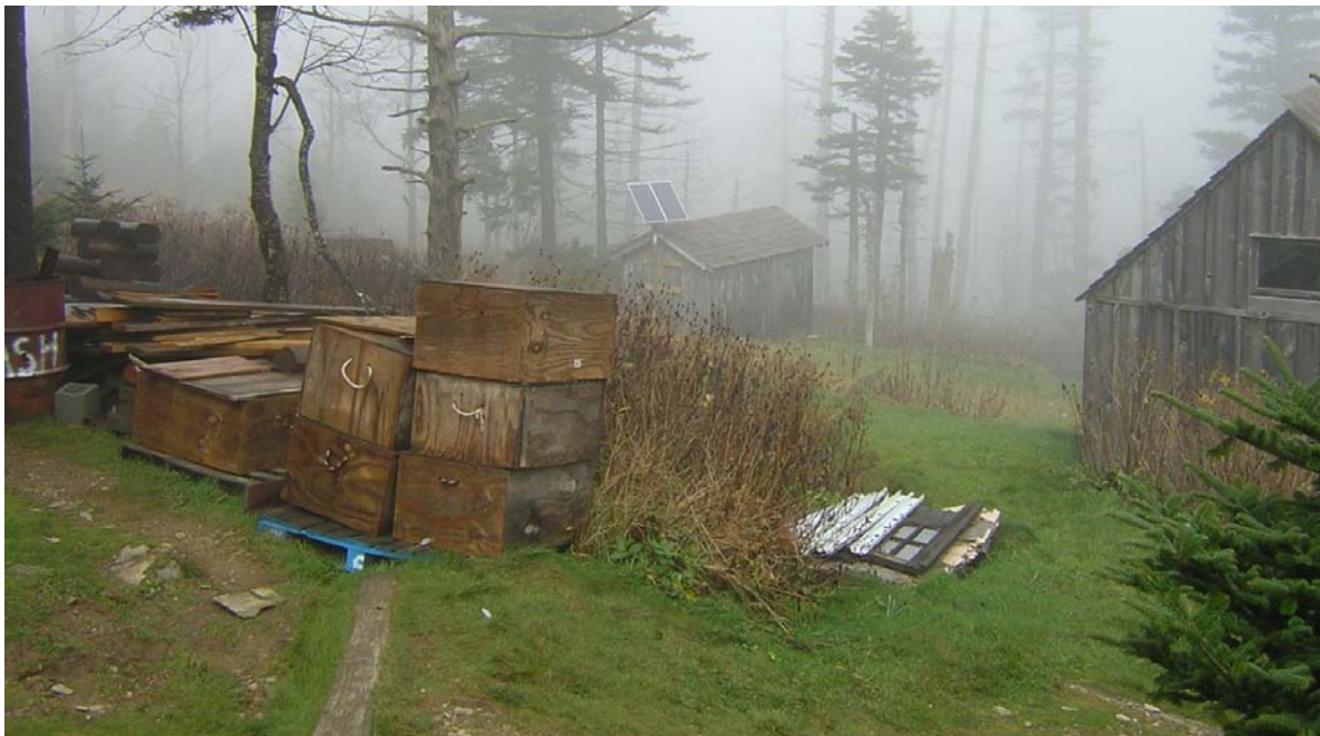
Figure 6.3 Pile of construction material beside woodshed. October 24, 2004 Photographer: William Shealy (author)
