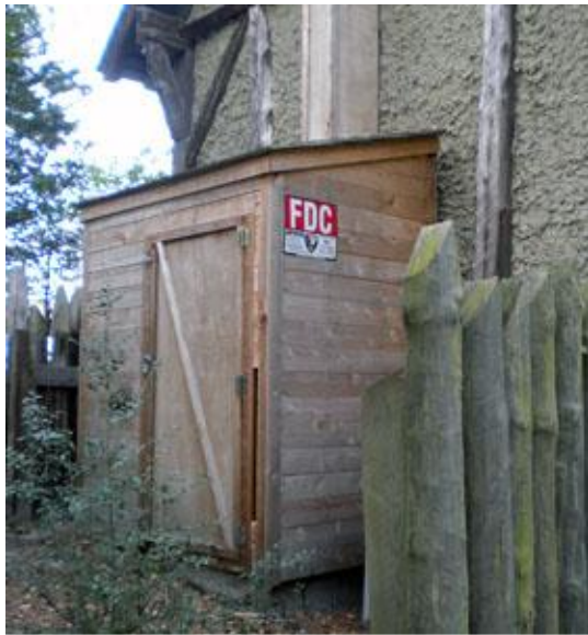
Figure 5.7: New Fire Sprinkler System
