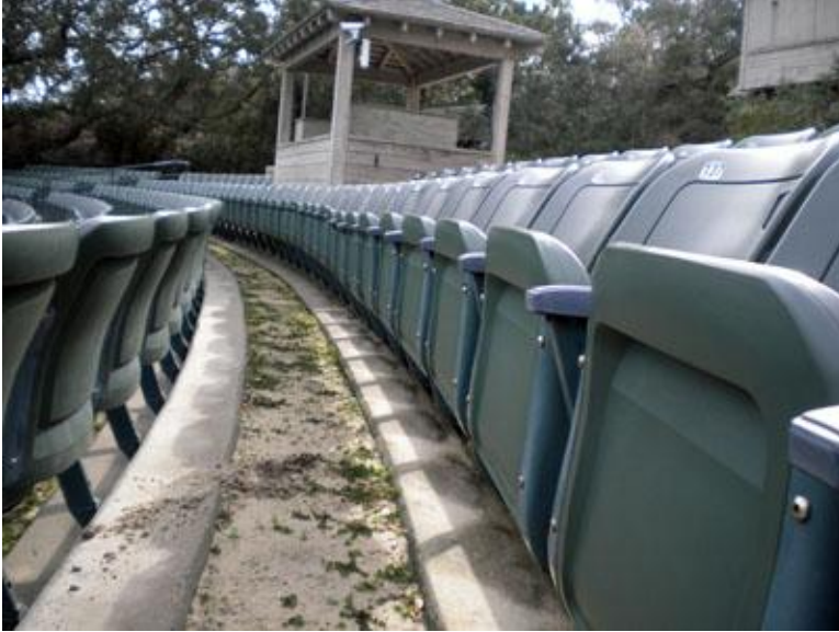
Figure 5.16: Sand Troughs Used for Stormwater Management
