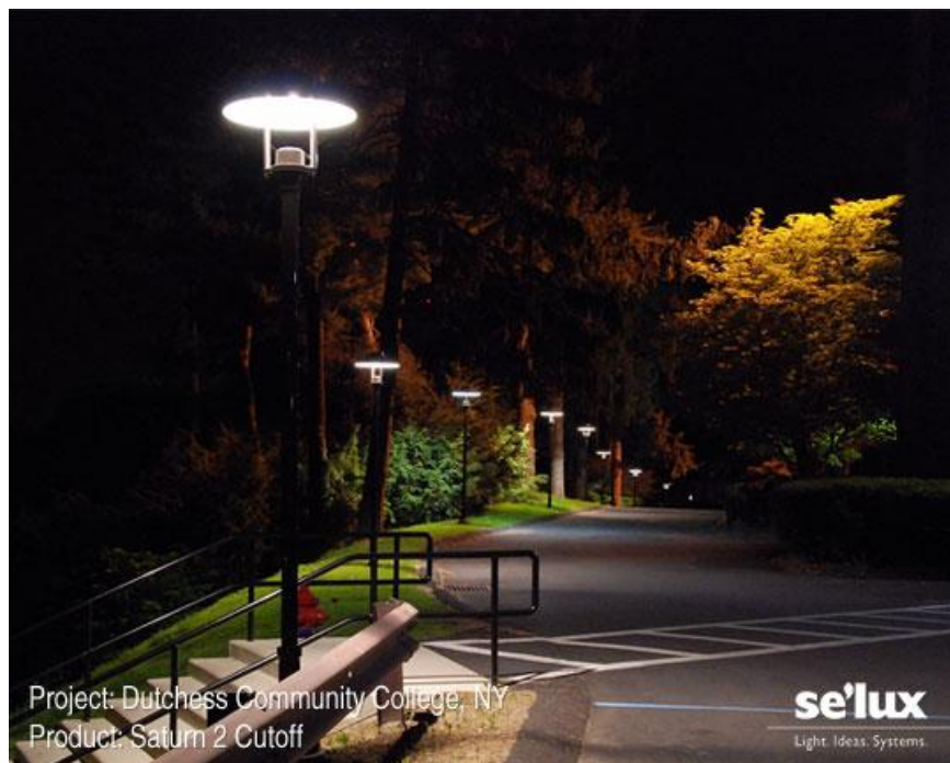
Figure 5.11 Selected full-cutoff pole-mounted lamp
