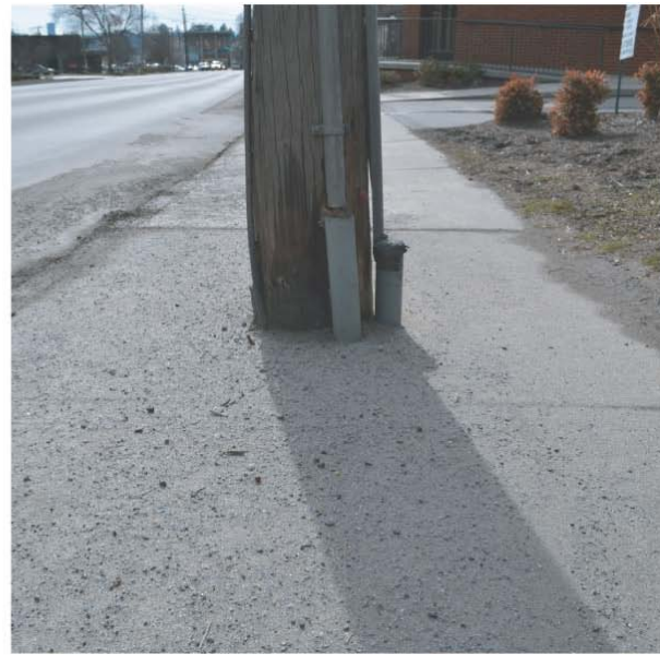
Photo D.4: Pedestrian Way Obstruction
