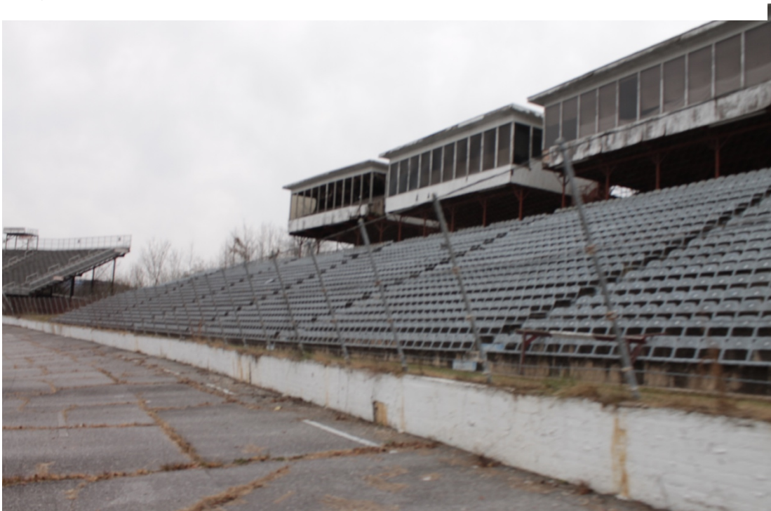
Figure 16. Front stretch suites and press boxes which are in overall poor condition. (Photo Credit Jacob Cook)
