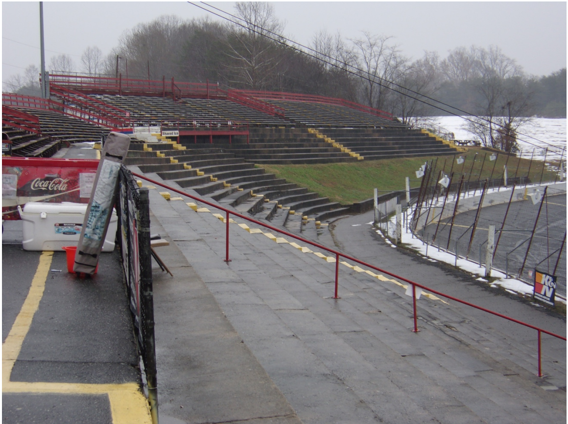
Figure 63. Front stretch and turn 4 concrete grandstands, with metal grandstand above concrete in turn 4.
