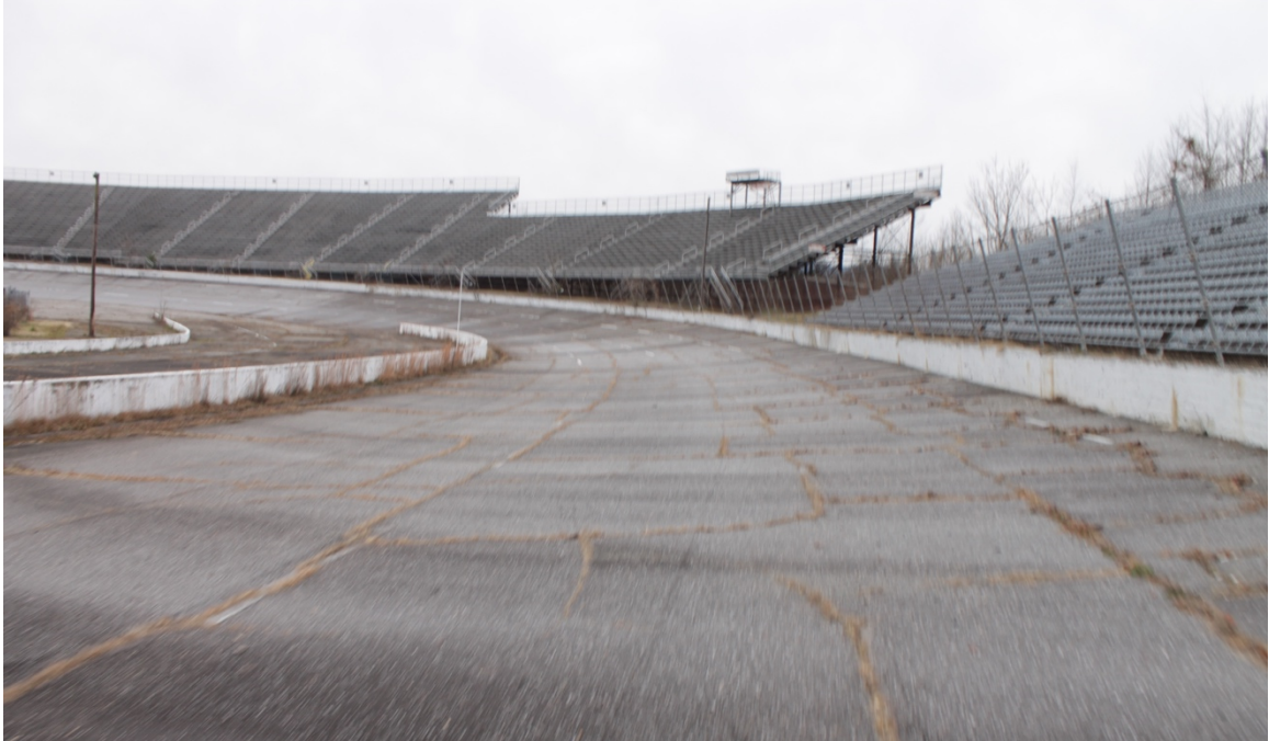
Figure 9. North Wilkesboro asphalt track surface still in overall good condition. (Photo Credit Jacob Cook).
