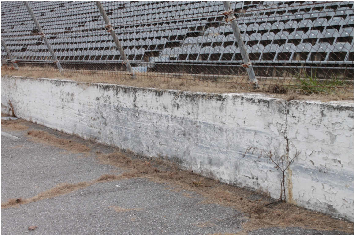
Figure 23. Close-up of outside wall, board forms are visible. (Photo Credit Jacob Cook)
