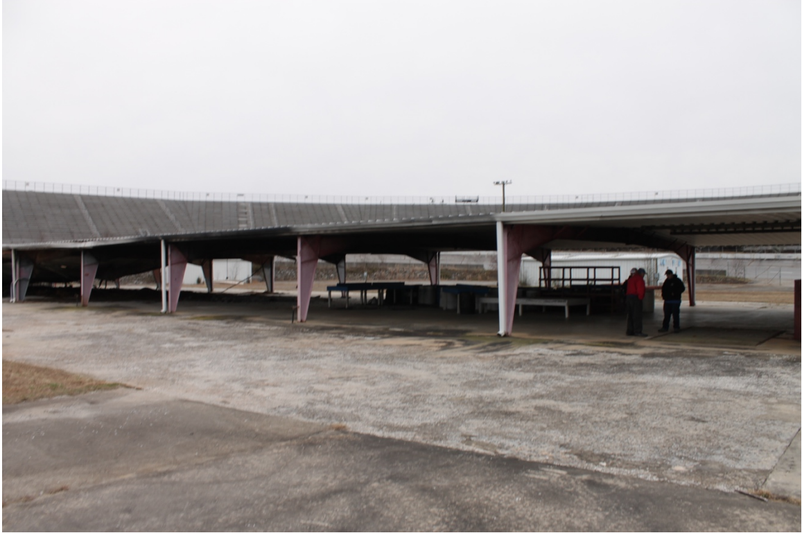
Figure 22. North elevation of garage which has sever fire damage. (Photo Credit Jacob Cook)
