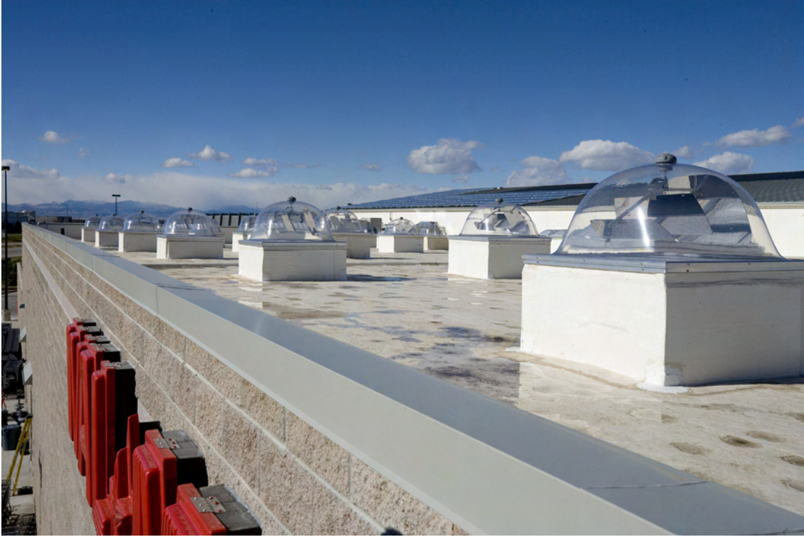
Figure 5.7: Active skylights and white membrane roofing at Aurora, CO. 347
