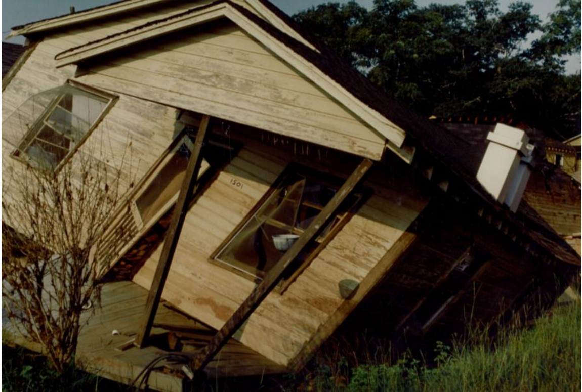
Figure 22. Dilapidated house after flood damage. 155
