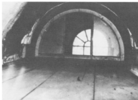
Figure 4.5 Lunette windows installed in the attic. (Source “An Early Victorian Passive Solar System”)
