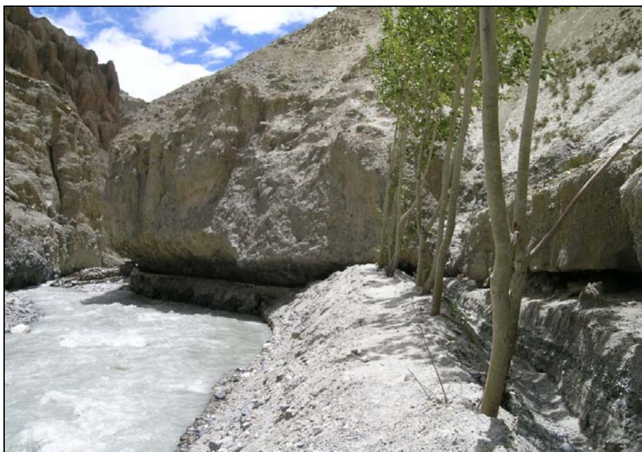
Figure 5.12 A section of the head-work of the upper canal along the Mustang Khola
