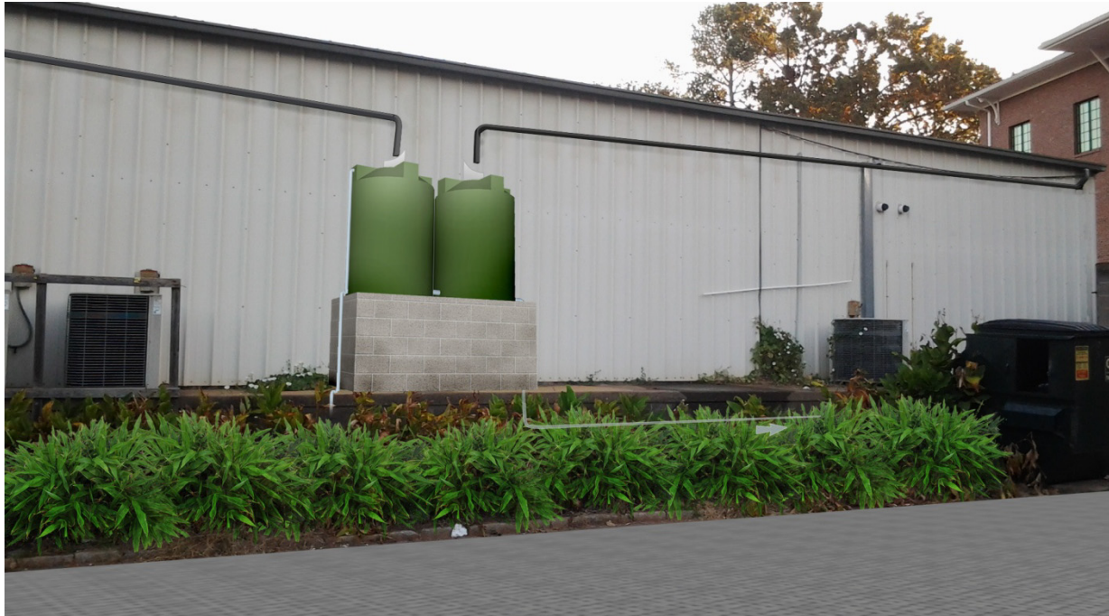
Figure 5.12 - Elevated cisterns behind Jittery Joe's for water feature in outdoor seating area
