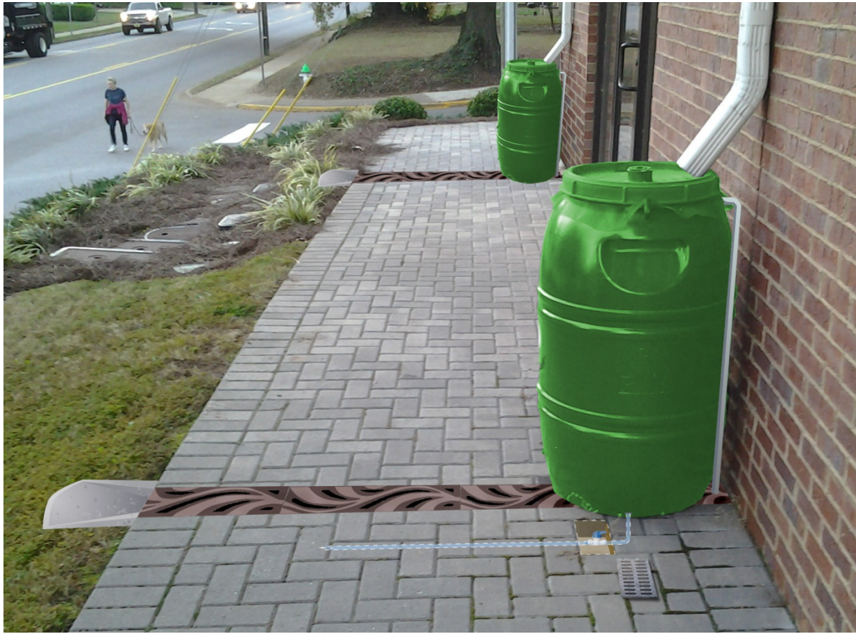
Figure 5.18 - Drain-delay rain barrels with overflow and drip hose connection
