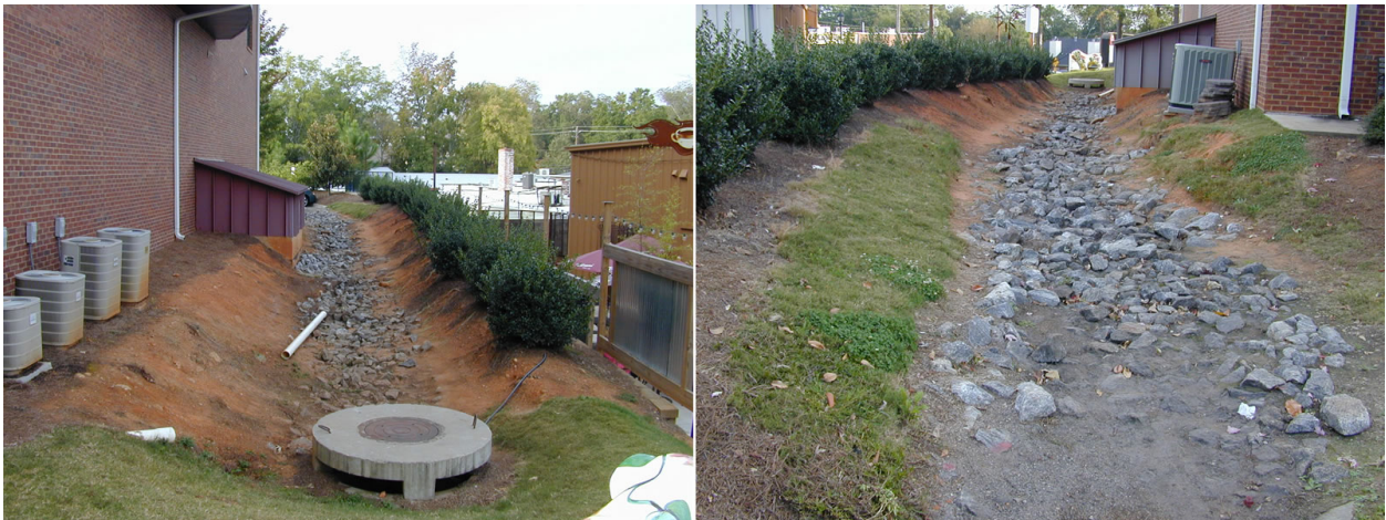
Figure 4.4 - Two views of a rock swale and weir that handles all drainage from mixed-use Building "D" parking
