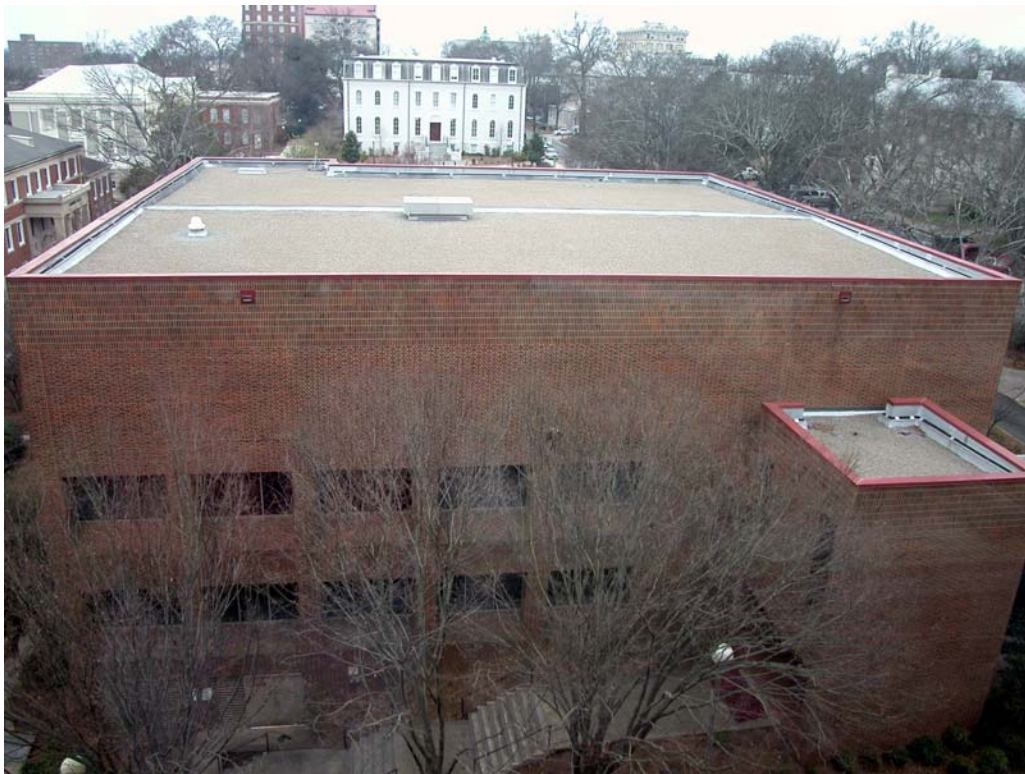
Figure 7.3 View north from the 5 th floor, Caldwell Hall, onto the law school library annex rooftop
