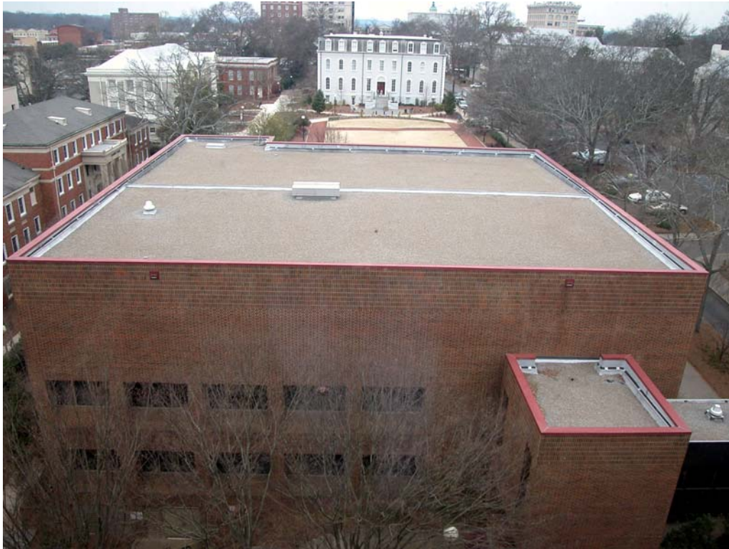
Figure 7.4 View north from the 6 th floor, Caldwell Hall, onto the law school library annex rooftop
